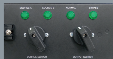
■ ITS Maintenance Switch
